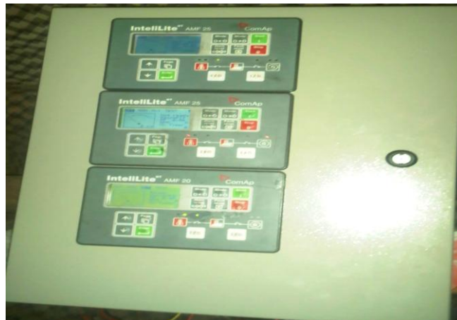
Fig12. Casing for the ACS
