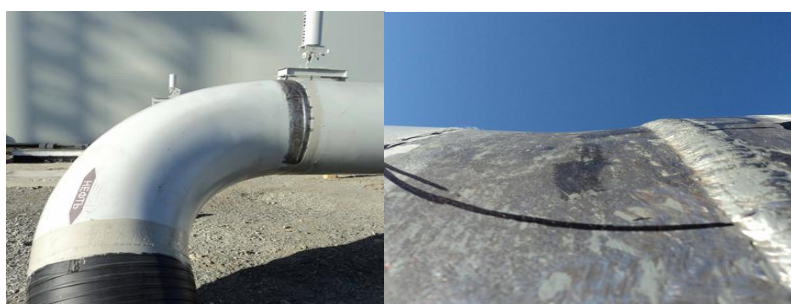
Fig. 9. Pipe joint with defect of "dent" type.
