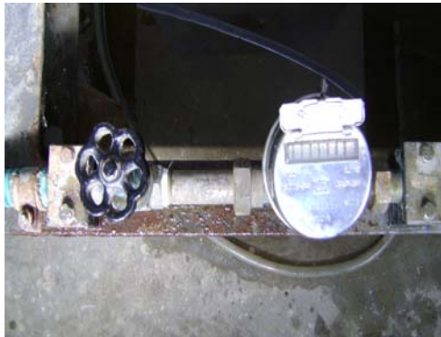
Figure7. Flow meter with gate valve
